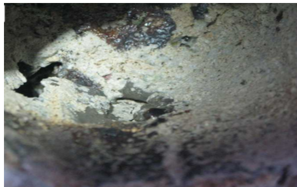
Figure 2.Boiler damage due to soot
